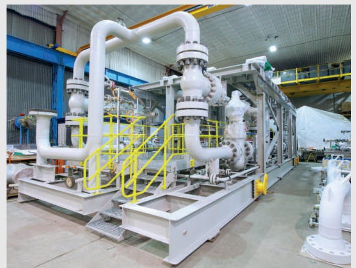
Completed Skid Package
